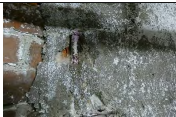
Incercarea ALC02 stalp - grosime strat beton carbonatat: 0-40mm
