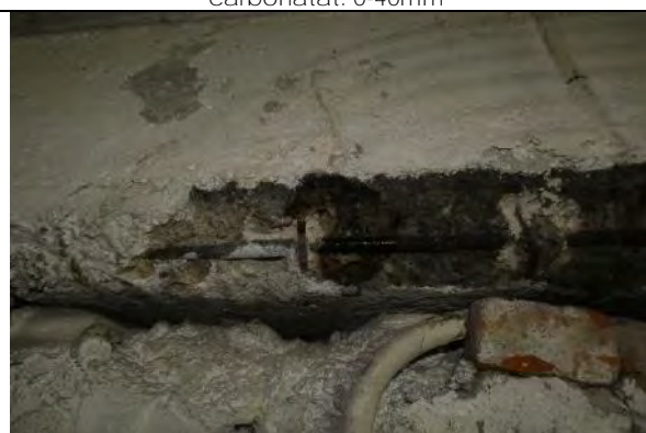
Incercarea ALC04 grinda - grosime strat beton carbonatat: 0-50mm
