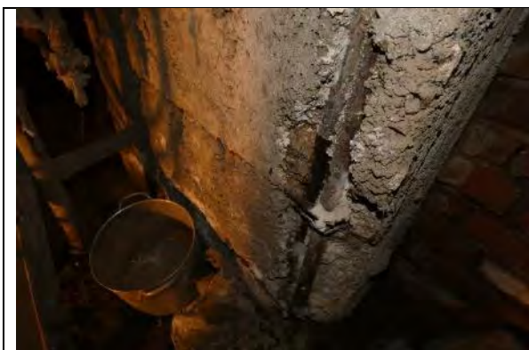
Incercarea ALC09 stalp - grosime strat beton carbonatat: 0-60mm
