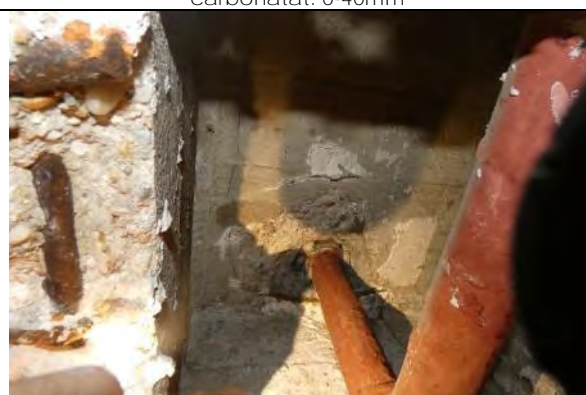
Incercarea ALC12 placa - grosime strat beton carbonatat: 0-30mm
