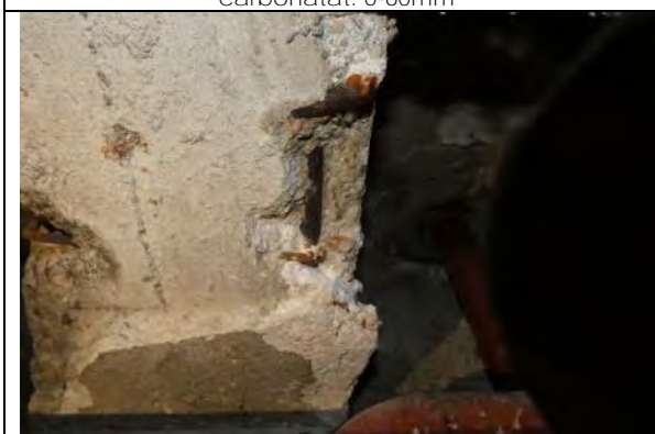
Incercarea ALC11 grinda - grosime strat beton carbonatat: 0-40mm
